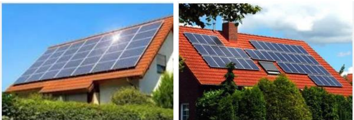
1-picture. An installed view of a solar power plant
