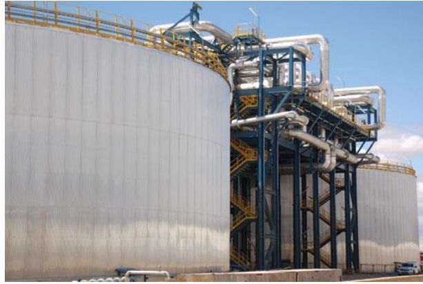
Figure-5.5.15. Two-tank molten salt system at the Andasol-3 solar thermal power plant (DLR has permission for this image).
