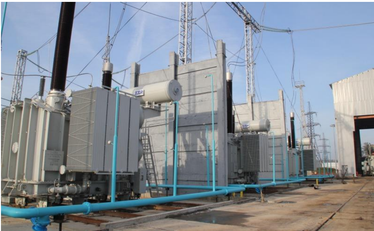
Figure 53. General view of single-phase autotransformers.
