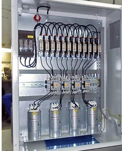
Figure 33. Capacitor bank for reactive power compensation
