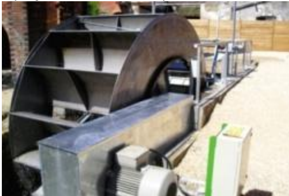
Figure 21. View of a micro hydropower plant with a windmill-type water turbine
