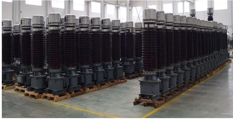
Figure 57. External view of a voltage transformer.
