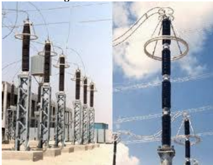
Figure 66. Arrester used in high-voltage networks.
