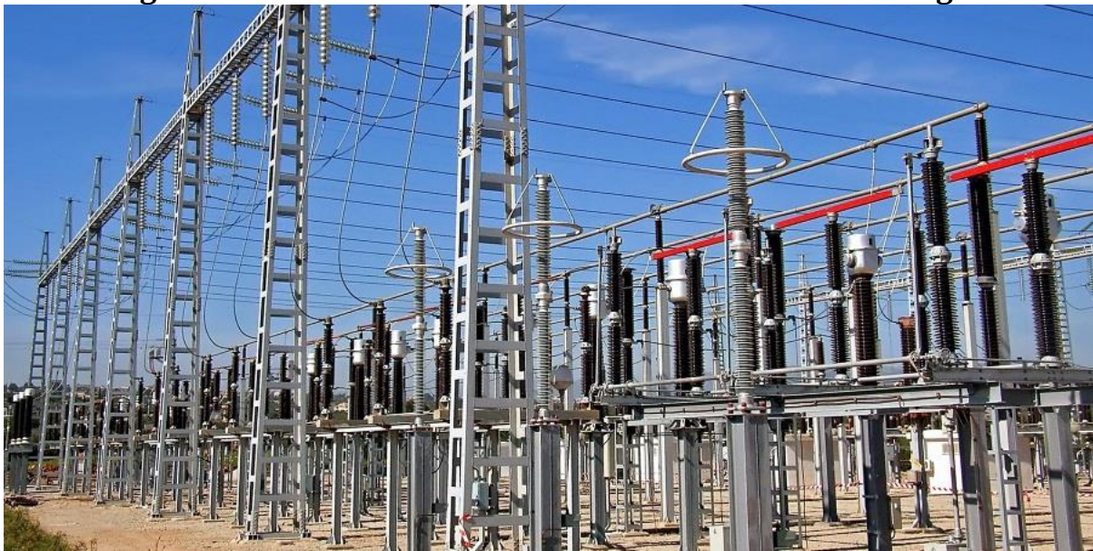
Figure 60. Open distribution devices used at high voltages.
