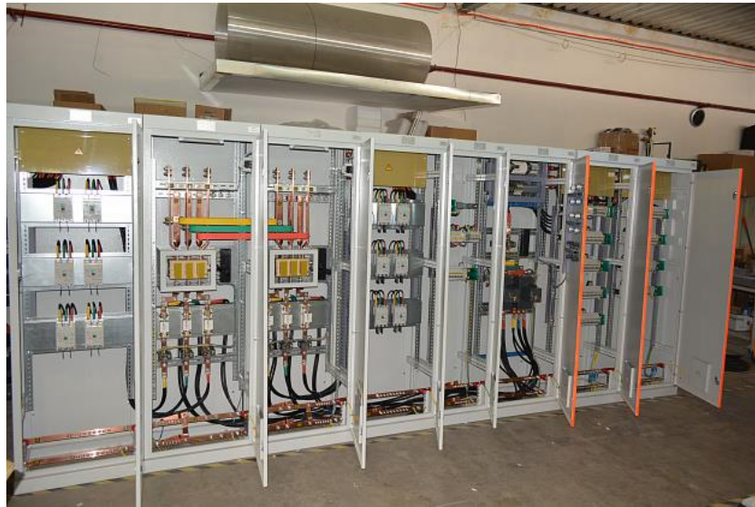
Figure 59. Closed distribution devices used at lower voltages.
