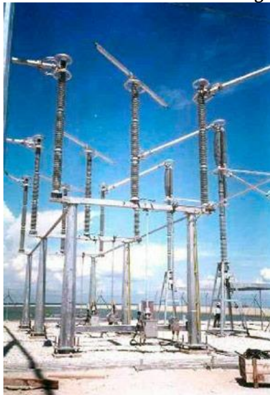
Figure 63. Disconnector used in high-voltage networks.
