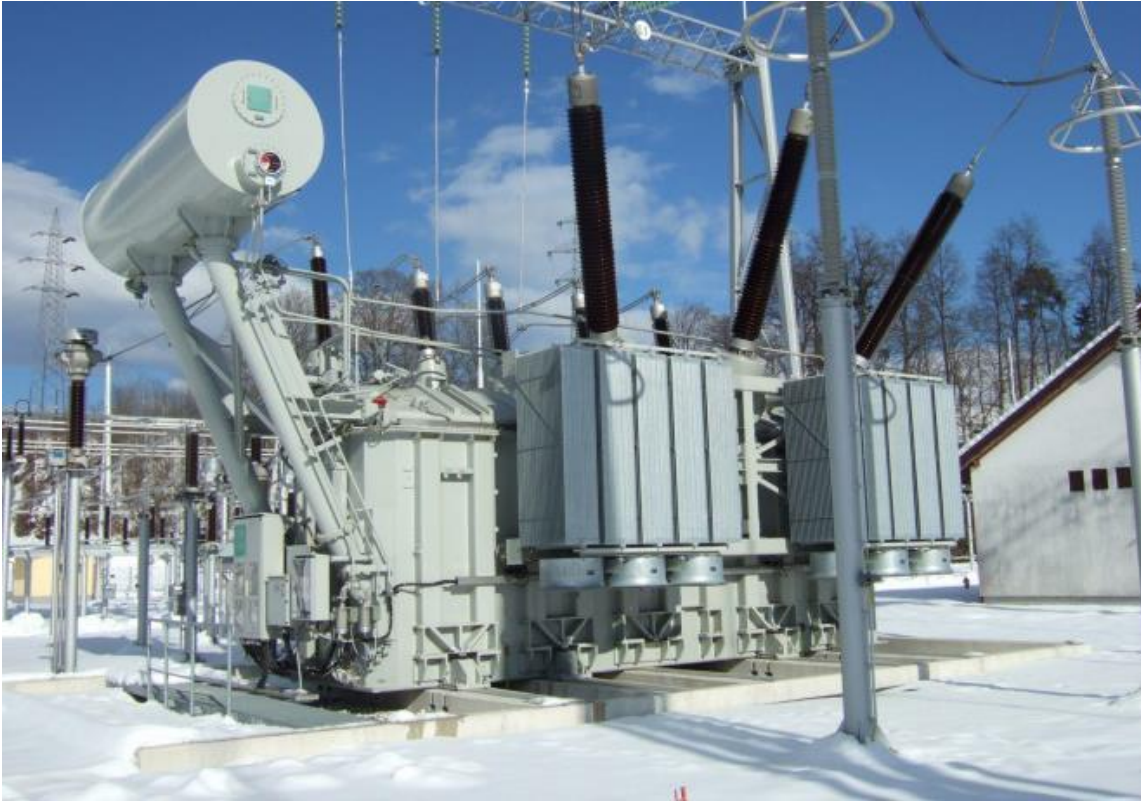
Figure 50. General view of power transformers.
