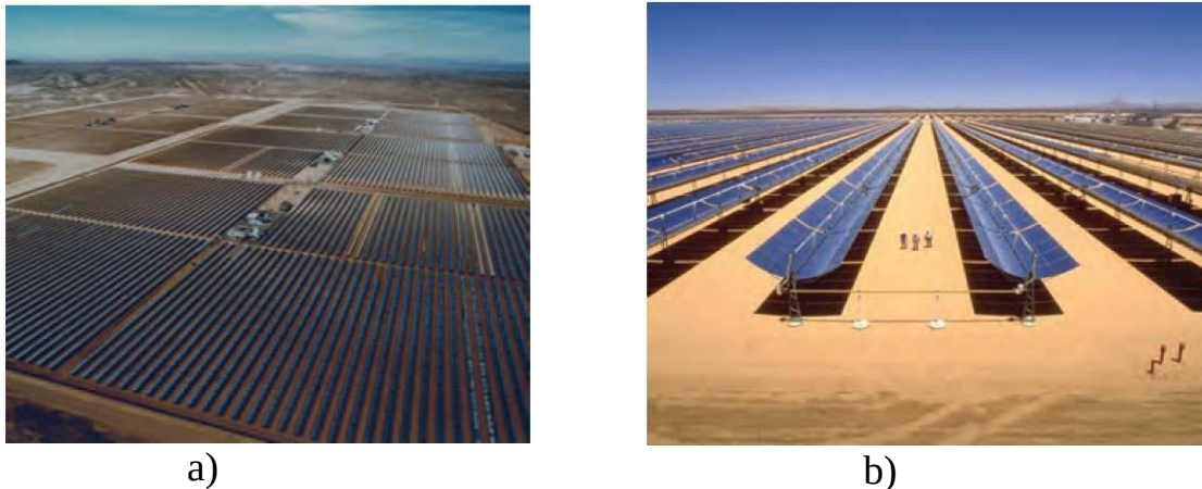
Figure 11-12. Arrangement of parabolic collectors at a solar thermal power plant in California, USA: a) general view; b) relative positioning of the collectors
