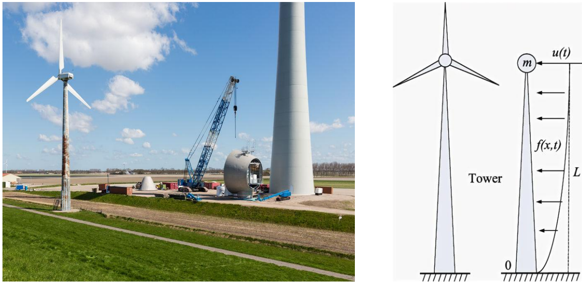
Figure 5.11. View of the wind power plant tower.
