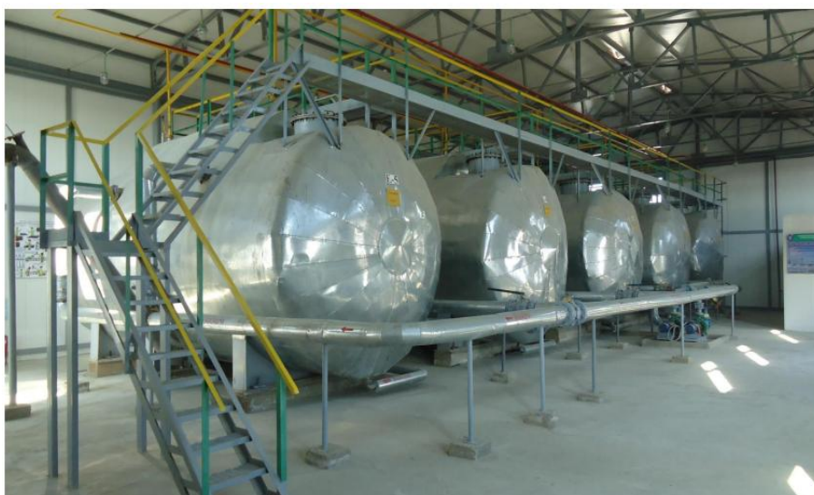
Figure 7.16. A biogas production unit operating on organic waste from the YOSHQ farm, affiliated with the Bukhara Oil Refinery, located in Qaravulbozor district of Bukhara Region.
