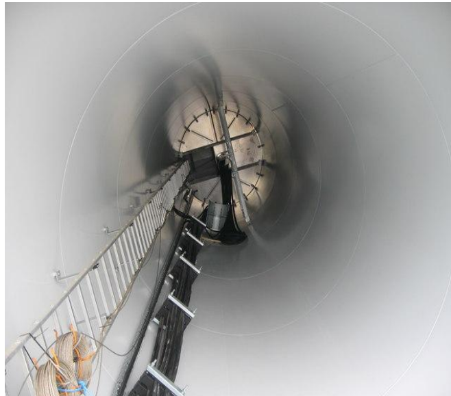
Figure 5.12. Internal view of a wind power plant tower.
