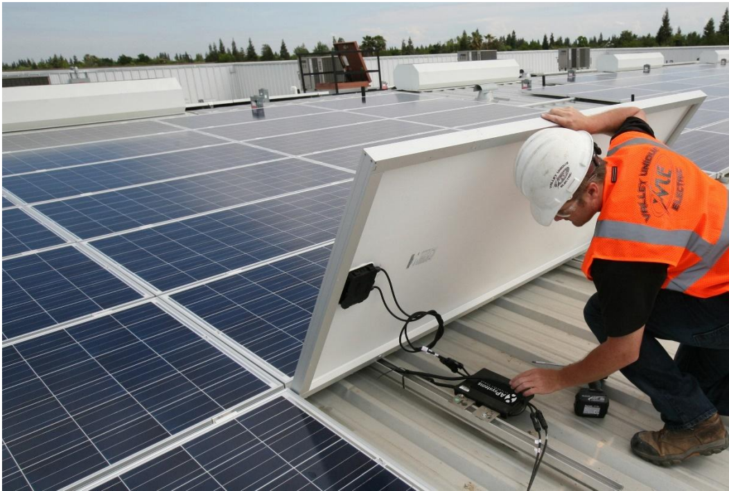
Figure 4.10 Microinverter mounted on the back of the solar panel
