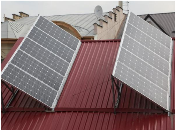
Figure 3.12 The position of the solar module device installed on the roof of the House
