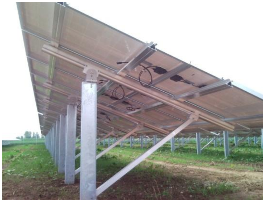
Figure 3.20. One-axis tracker solar power station
